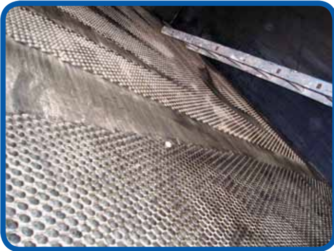
Condenser Power Station Treated with MEXEL 432
